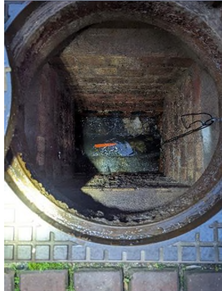
Photo: Partners for Urban Water
