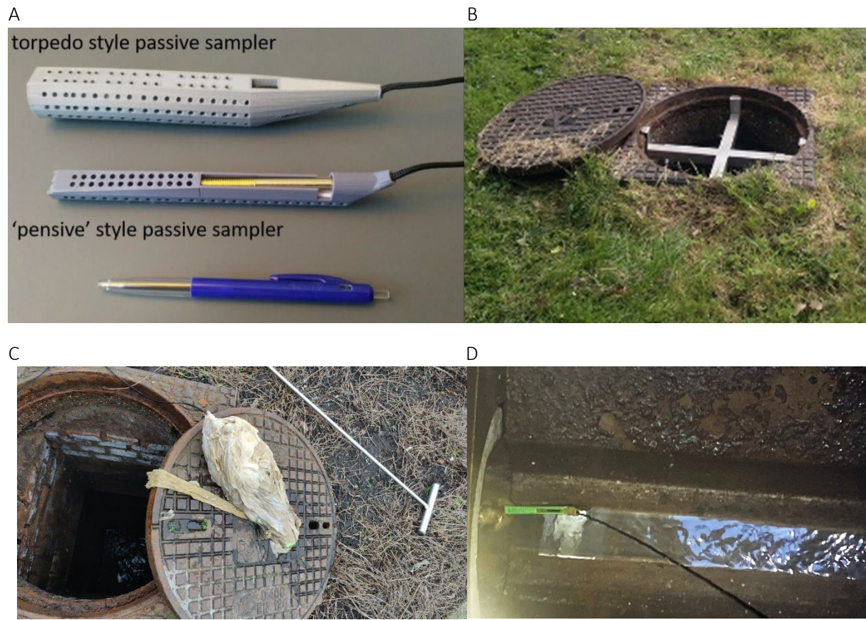
Figure S.1 Passive and pensive sampler (A) and installation in manhole (B) and of the quality control of the samplers, showing large amounts of wipes deposited on the sampler (C) or the sampler moved outside of the wastewater flow (D).
